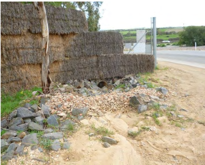
Plate 13: View of Front Entrance Surface Drainage system
