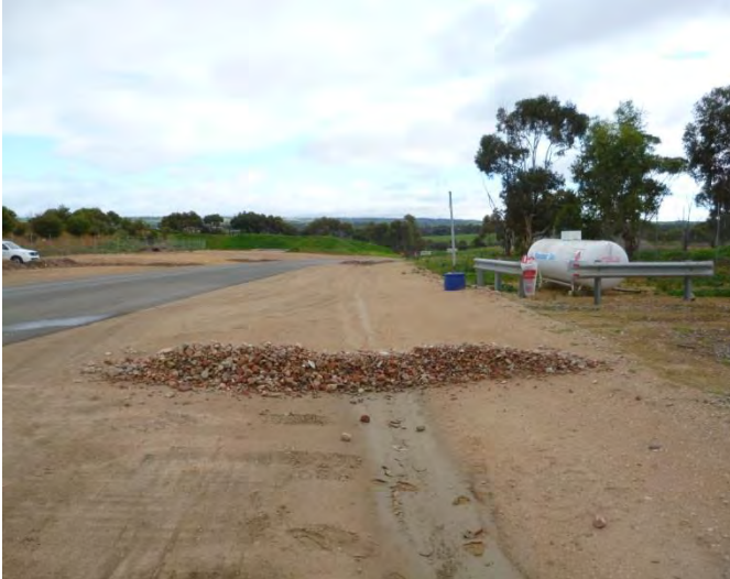
Plate 11: View of Silt traps at front entrance drive way, Eastern side
