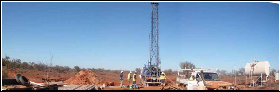
Plate 1 - Walsh Drilling constructing Challenger Production Observation Well 02 (CPOW02) next to Challenger Production Well (CPW02) (February, 2007)
