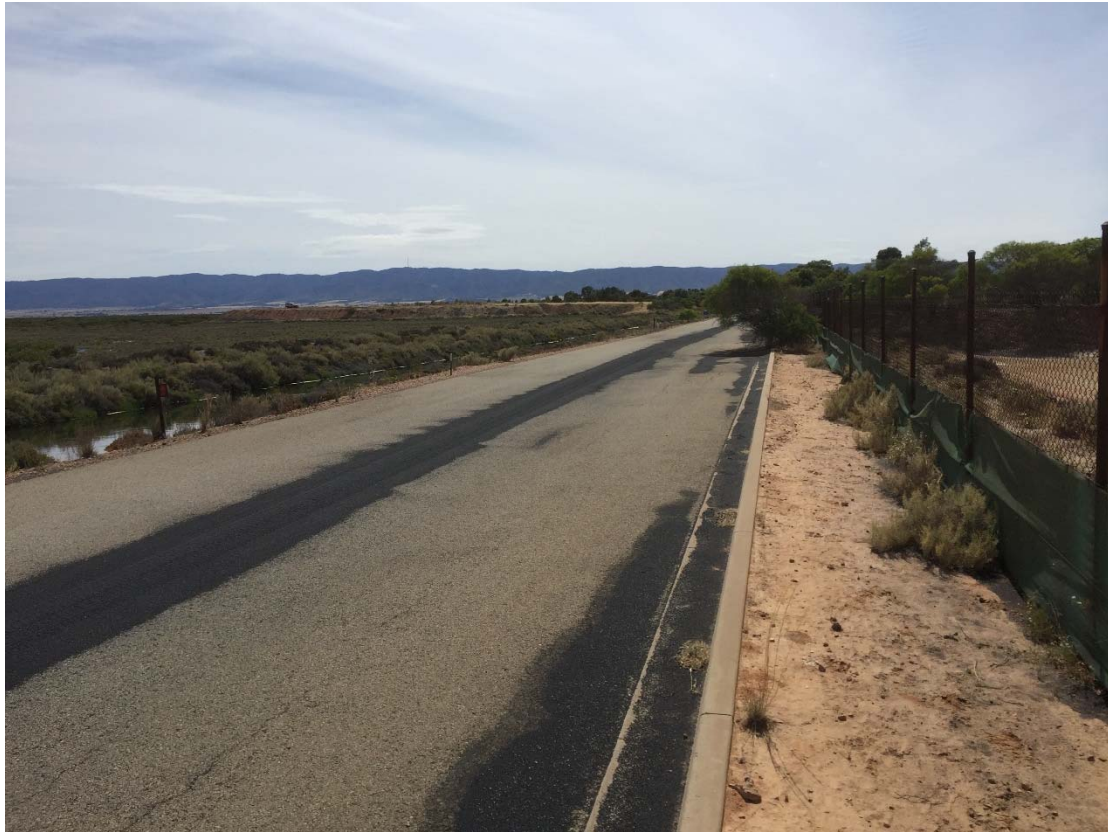
Figure 12 North road embankment looking east separates the tidal mudflats from the dams.
