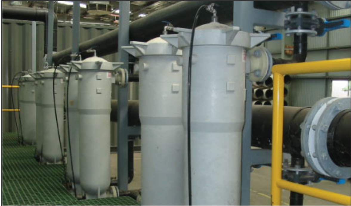
Plate 4.3 Filter skids used at Honeymoon mine
