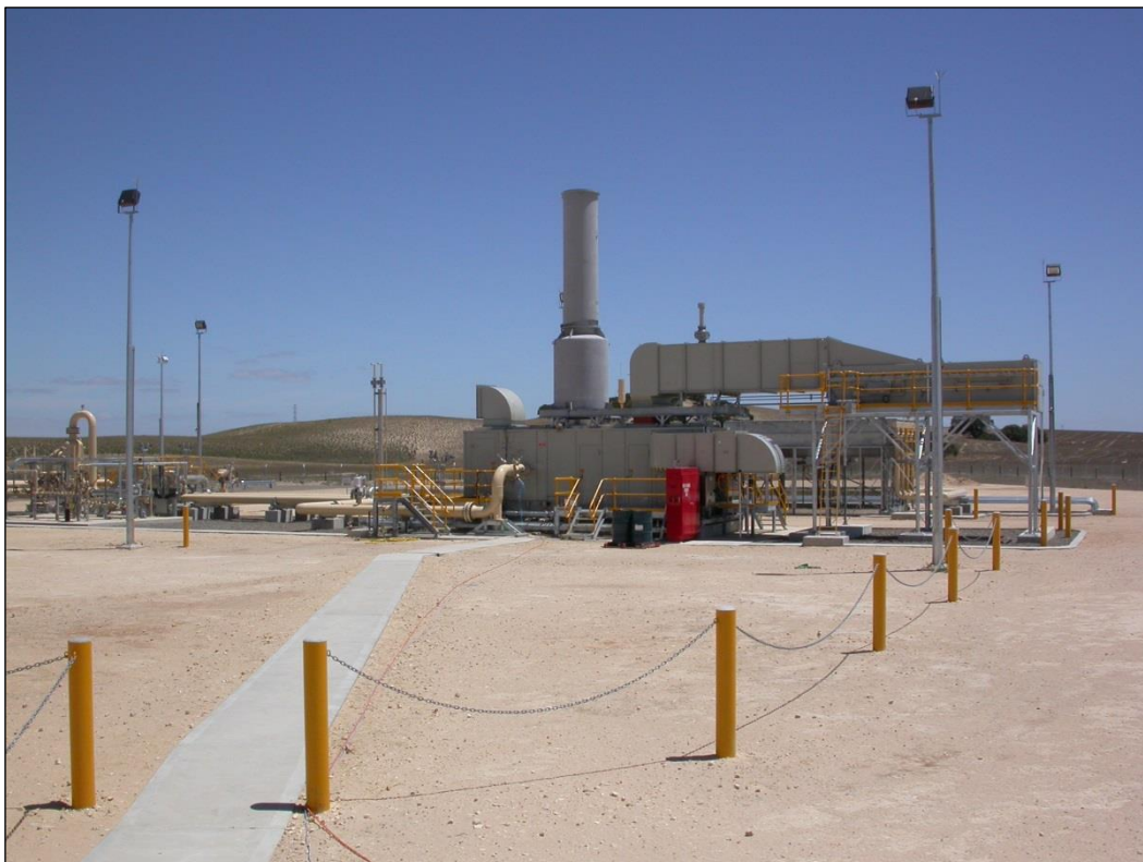
Plate 3-4: Coomandook Compressor Station
