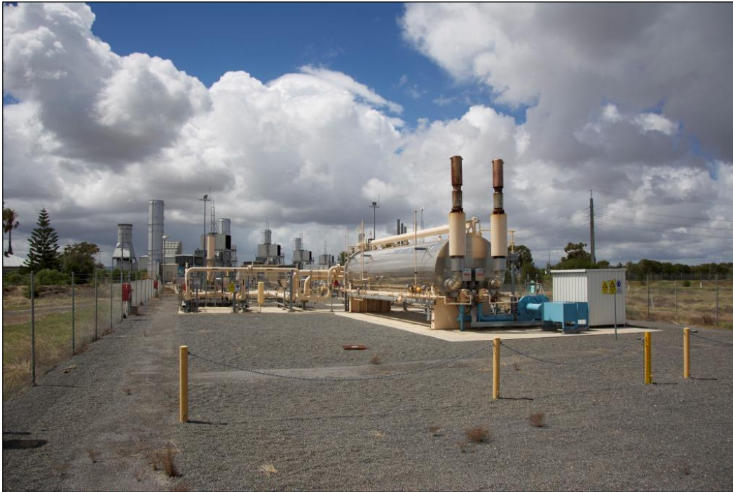
Plate 3-3: Quarantine Meter Station
