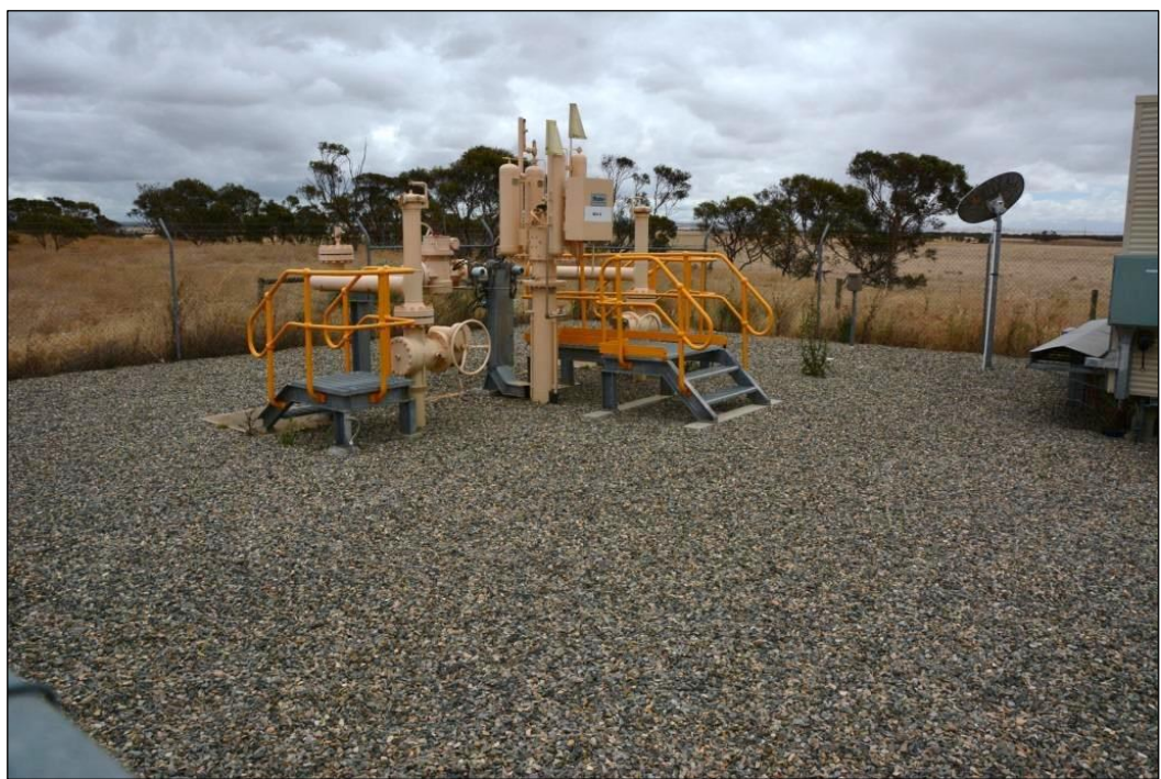
Plate 3-1: Pallamana Mainline Valve
