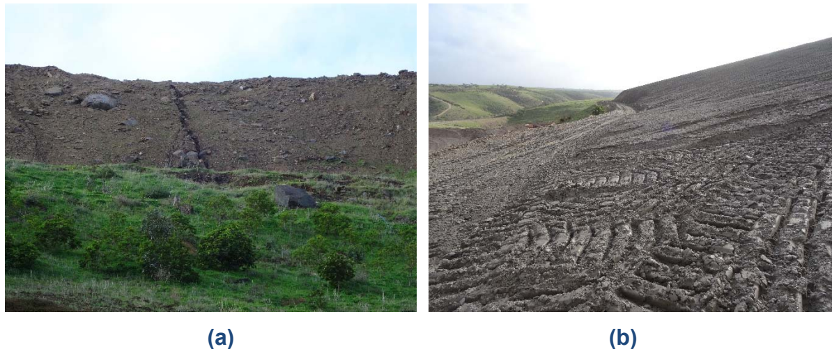
Figure 10 Reshaping and covering, showing: (a) unreshaped upper lift of TSF, and (b) reshaped IWL slope covered with NAF waste rock
