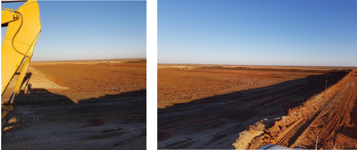
Figure 3-39: Compaction of the Trial Section of TSF-2 after Removal of Tailings Material
