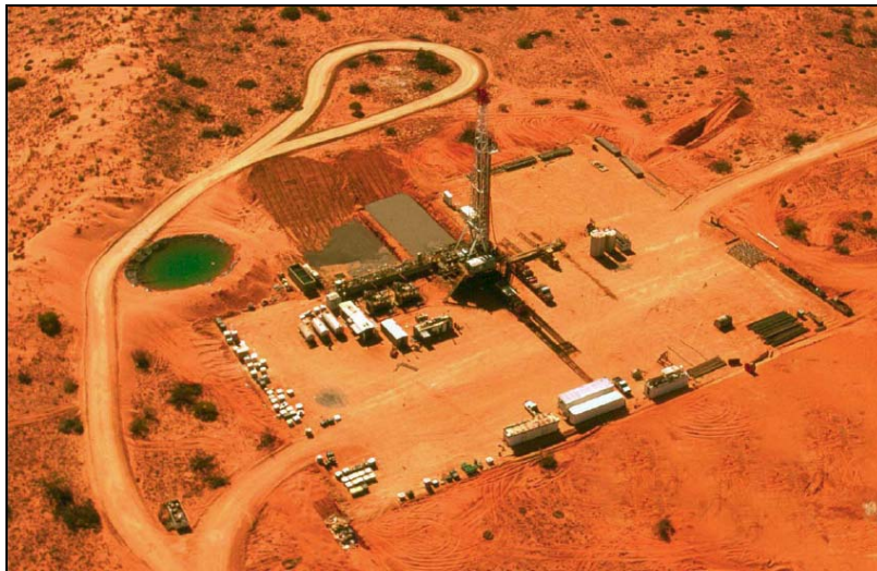
Plate 1: Petroleum drilling rig showing typical layout of well lease (Source: Santos 2003)
