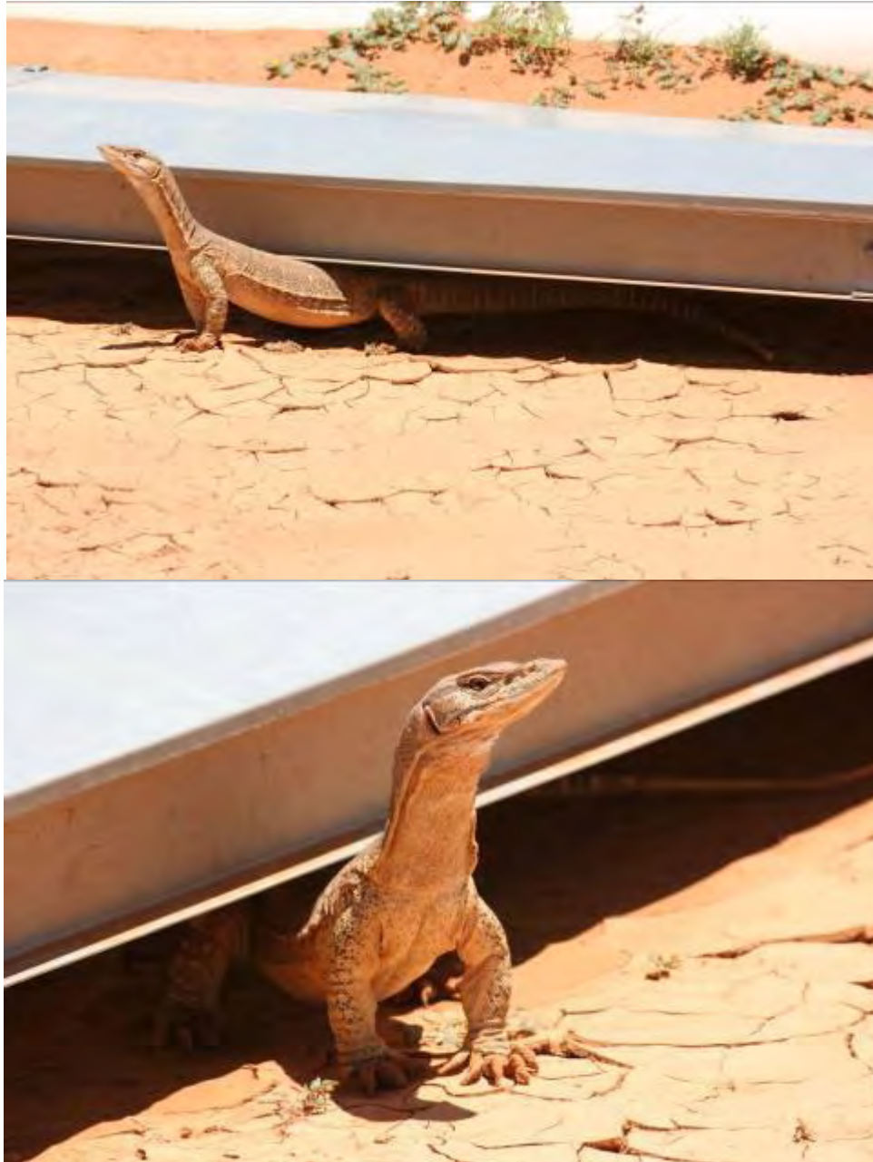
Plate 2-1: A goanna ( Varanus gouldii ) emerging from beneath a cable tray that runs from the processing plant to the wellfields alongside the trunklines
