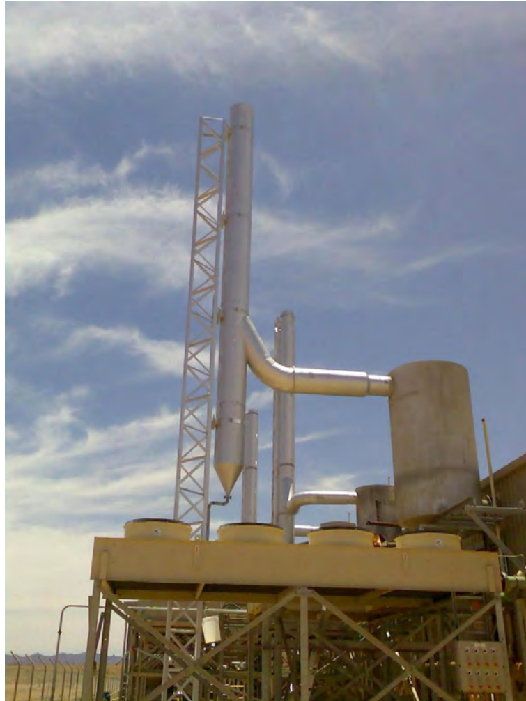
Plate 3-7: Gas fired generator exhaust stacks installed and commissioned
