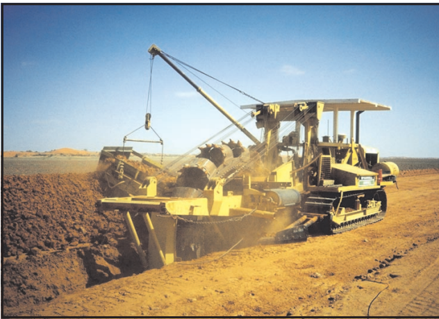
Trenching in preparation for laying of South-West Queensland gas pipeline to South Australia, 80 km northeast of Moomba, April 1992. (Photo 40368)
