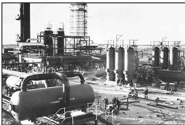
The Moomba Natural Gas Processing Plant under construction in September 1969. (Photo N019880)
