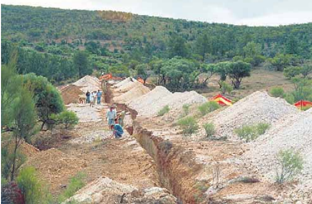
Trenching at the headwaters of Calabrinda Creek where abundant diamond indicator minerals were found in sediments thought to be sandy tuff. (Photo 46793)
