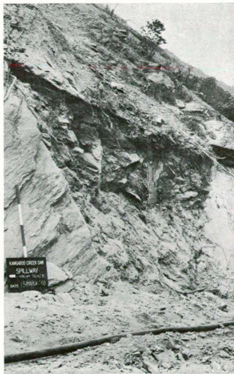
Fig. 18. Soil mass of rock fragments and clay, filling a V-shaped gully formed by sliding of wedge mass bounded by Set (1) and Set (2) joints; central part of spillway excavation.
