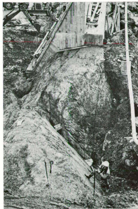
Fig. 19. V-shaped gully formed by sliding along Set (1) and Set (2) seams; spillway channel, north wall—foundation for block LH.
