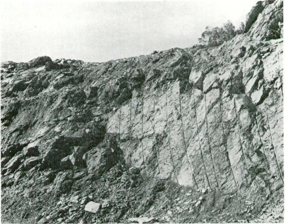
Fig. 86. Part of batter for quarry No. 1, bench 3. Pre-split is almost planar except towards the top of the batter where some overbreak has occurred.
