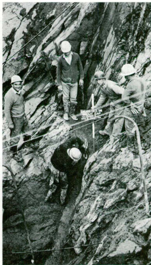
Fig. 33. Foundation for grout cap with infilled clay seam 5 cm wide after dental treatment.
