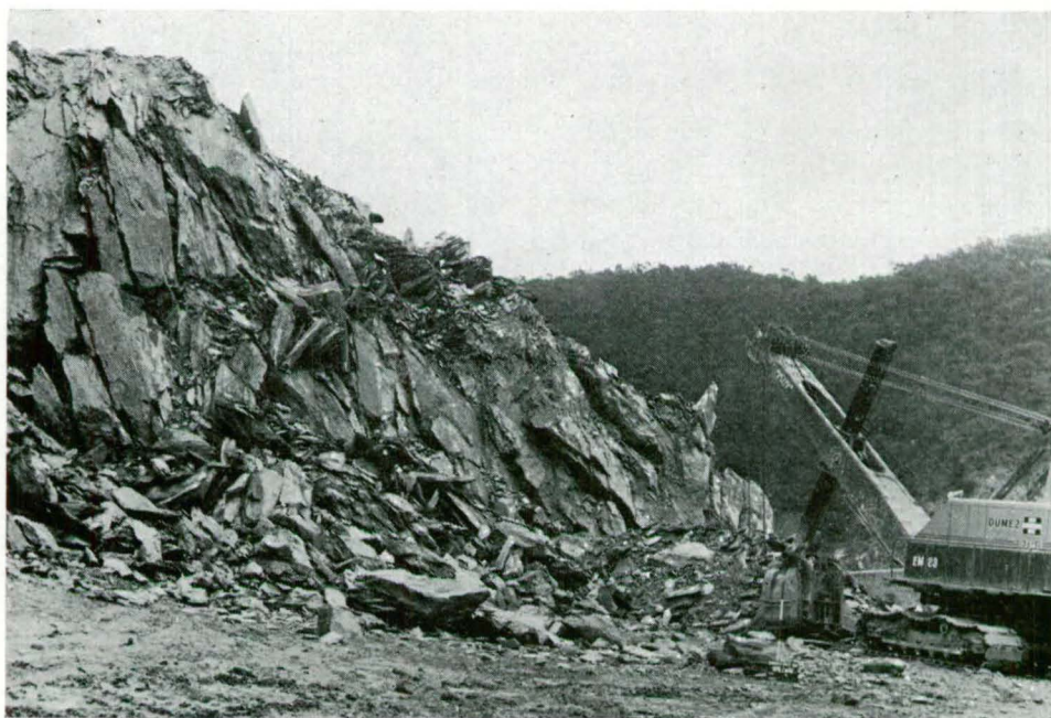
Fig. 54. Face of spillway excavation, bench 4. Primary blasting and some secondary blasting (foreground) have produced highly flaky fragments of the weak schist.
