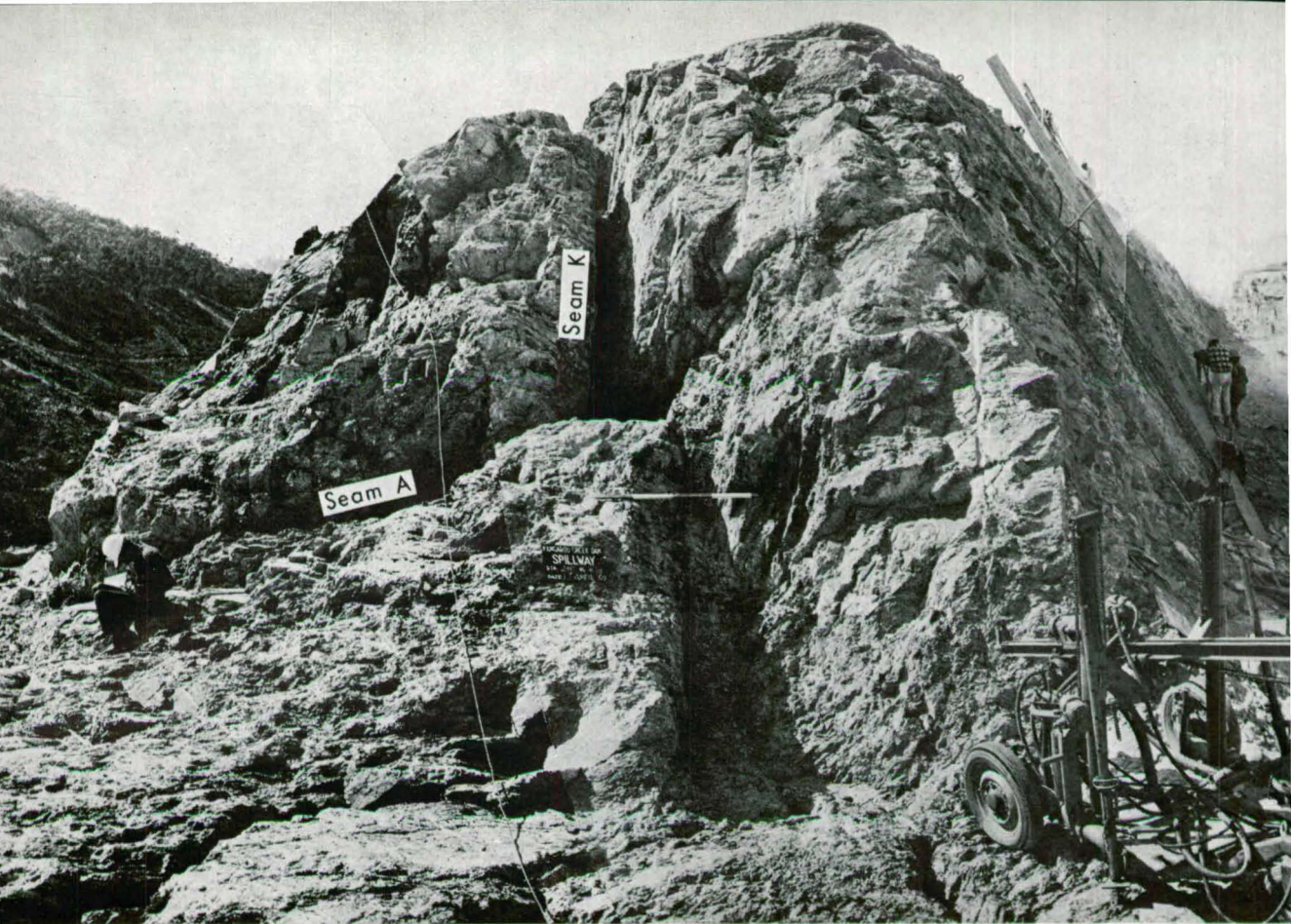
Fig. 46. Initial excavation for spillway block LE showing disturbed rock containing thick seams of infilled clay (seams K and A).
