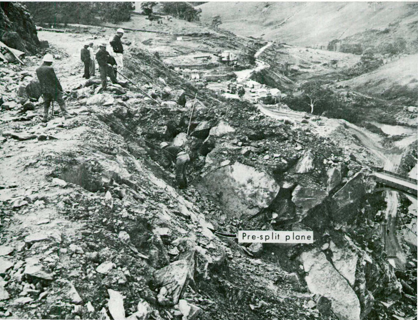
Fig. 68. Loose rock remaining on pre-split batter after blasting of knob on right abutment.
