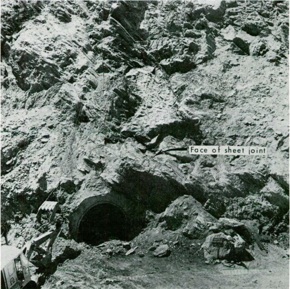
Fig. 52. Lower part of intake structure excavation showing pre-split floor, underlain by sheet joint.
