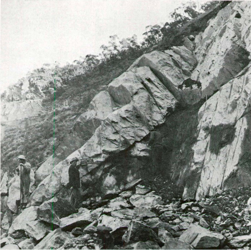
Fig. 70. Partly open sheet joints exposed in the downstream wall of the access shaft open cut.
