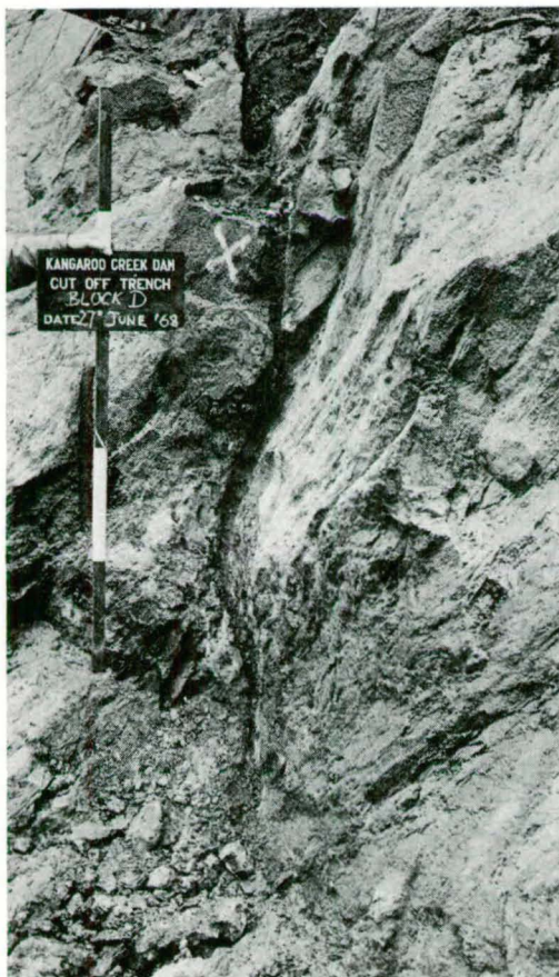
Fig. 32. Foundation for grout cap with infilled clay seam 5 cm wide before dental treatment.
