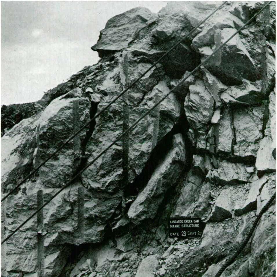
Fig. 51. Sheet joints gaping open to 20 cm in upper part of intake structure excavation, downstream wall.
