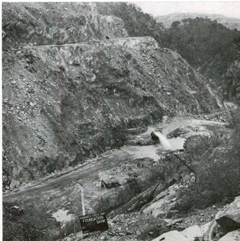
Fig. 22. Left abutment after removal by D8 bulldozer of soil materials up to 20 feet thick, which occurred beneath a shallow gully up to 200 feet wide.
