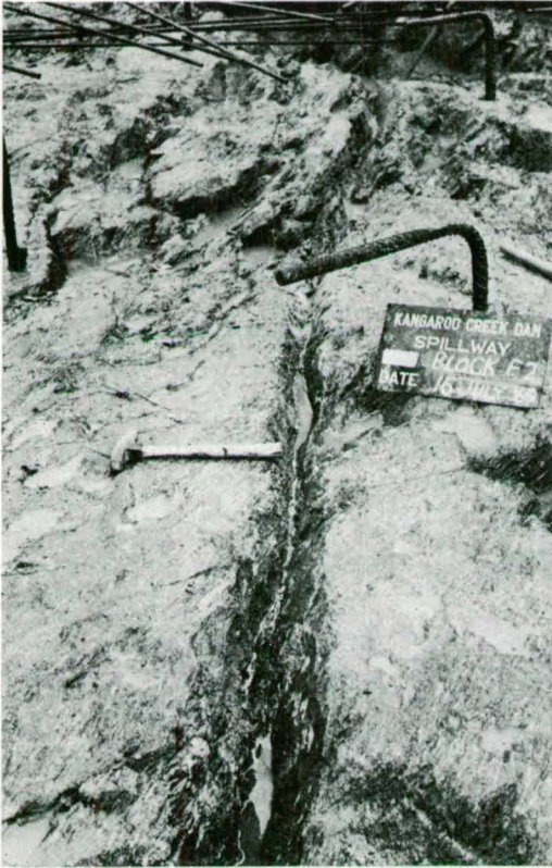
Fig. 42. Narrow crushed seam exposed in the floor of the spillway channel excavation before wet seam treatment.
