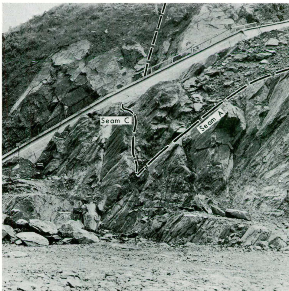
Fig. 74. Base of wedge mass No. 1 exposed in embankment foundation downstream of grout cap, block C.
