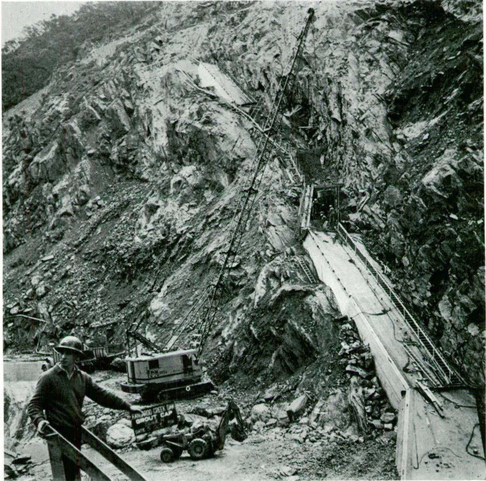
Fig. 28. Construction of grout cap on right bank. Blocks F, G and K are complete. Pouring of block H in progress.
