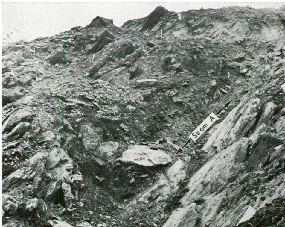
Fig. 73. Early stage in excavation for grout cap, block B through soil and disturbed rock—part of wedge mass No. 1.
