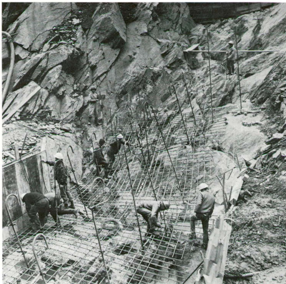
Fig. 29. Erection of lower layer of reinforcing steel mesh in grout cap, block E.
