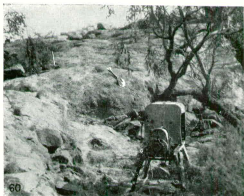
FIG. 60—MINDAMEREKA HILL URANIUM PROSPECT Boring plant site P.P.I.—Peg marks main area of radioactivity, and borehole collar is indicated by a shovel
